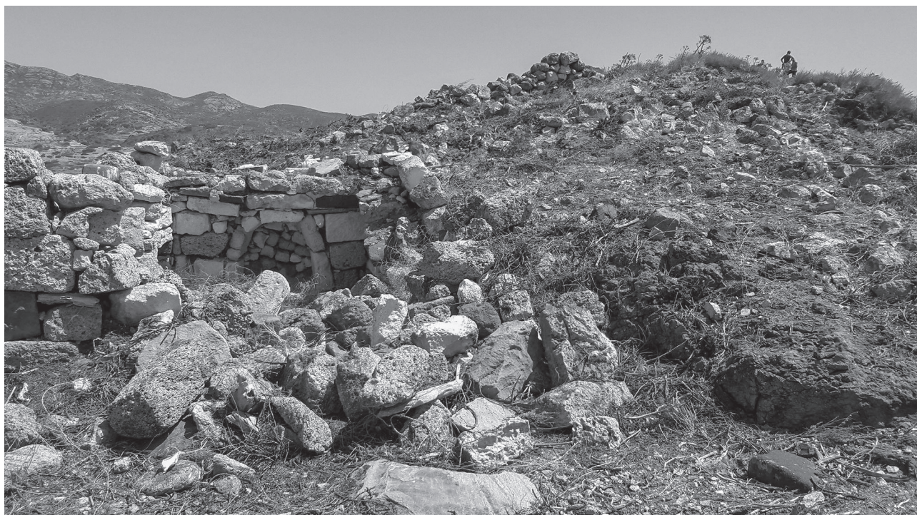
Fig. 5a - The post-Byzantine church at the western end of the islet of Agios Andreas. In the foreground elements of the collapse of the facade and the vaulted ceiling (Photo C. Di Nicuolo)
