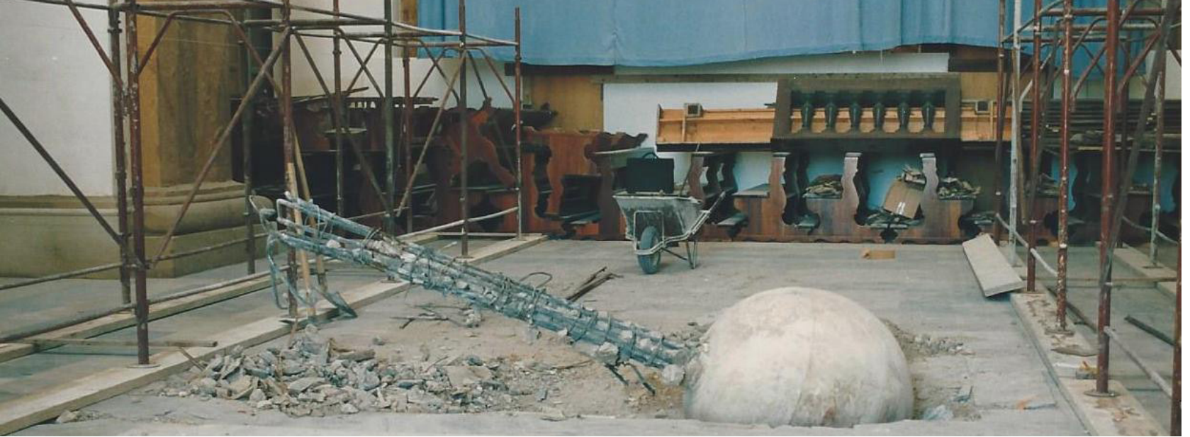
Fig. 8-10: Disconnection of the masonry following the detachment of the sphere; Hole in the cover caused by detachment and falling of the sphere; Stone globe with cross in the central nave after falling from the bell tower [Berenato 1994].
